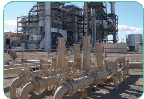
Figure 10 – Slam Shut and Fast-Acting Monitor Regulators Natural Gas Fired Power Plants (Power Generation Industry)
