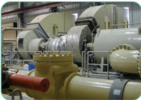
Figure 9 – Surge Control Valves Centrifugal Natural Gas Compressors (Natural Gas Transmission Industry)
