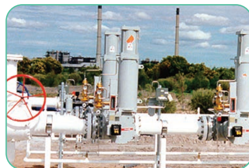
Figure 13 – Becker RPSR Actuated Control Valves in Power Plant
